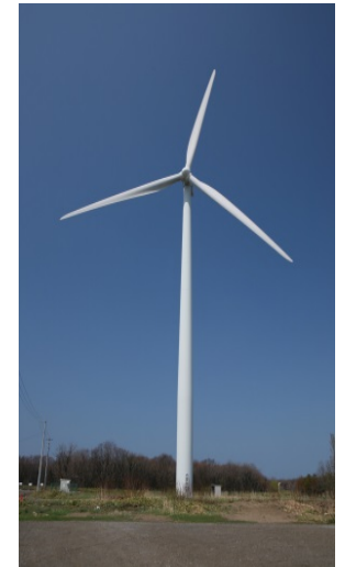
Figure 3b Wind turbines used for wind power generation. http://sozai-free.com/sozai/01541.html
